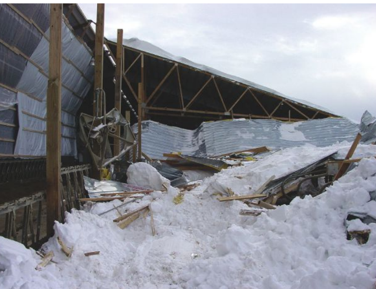
Cyril Myren and his son Todd were injured during the above roof collapse, which was attributed to a lack of diagonal bracing on the continuous lateral bracing used to keep truss web members from buckling.
