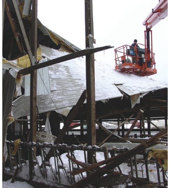
Workers remove roof sections that collapsed due to improperly braced trusses.
