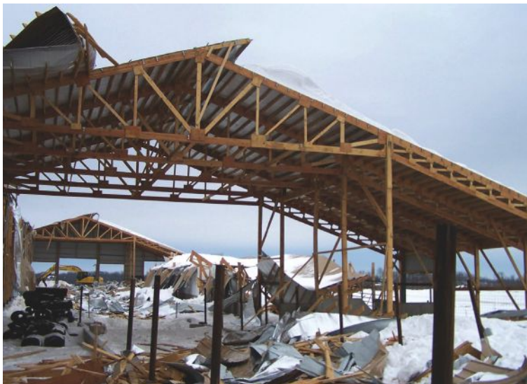
All but the endwalls and a middle section of this non-engineered building failed when columns buckled under, again, the first snow load. Subsequent calculations showed columns with a near-zero axial design load capacity.
