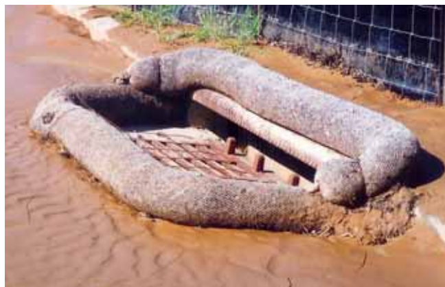
Filtrex Inlet Protection system captures runoff pollutants before entering storm sewer system.
